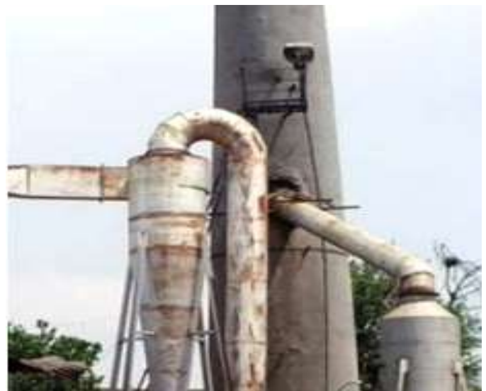
Rolling Mill with APCD
